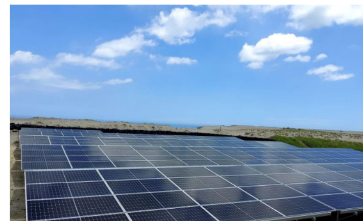
[WWB Kamisu Solar Power Plant] An example of an operational project developed in Kamisu, Ibaraki Prefecture.
