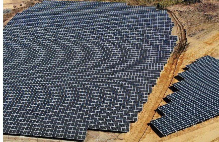
Hanabatake Solar Power Plant (Gunma Prefecture) / (DC): Approx. 3.6MW
