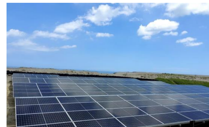
[WWB Kamisu Solar Power Plant]
