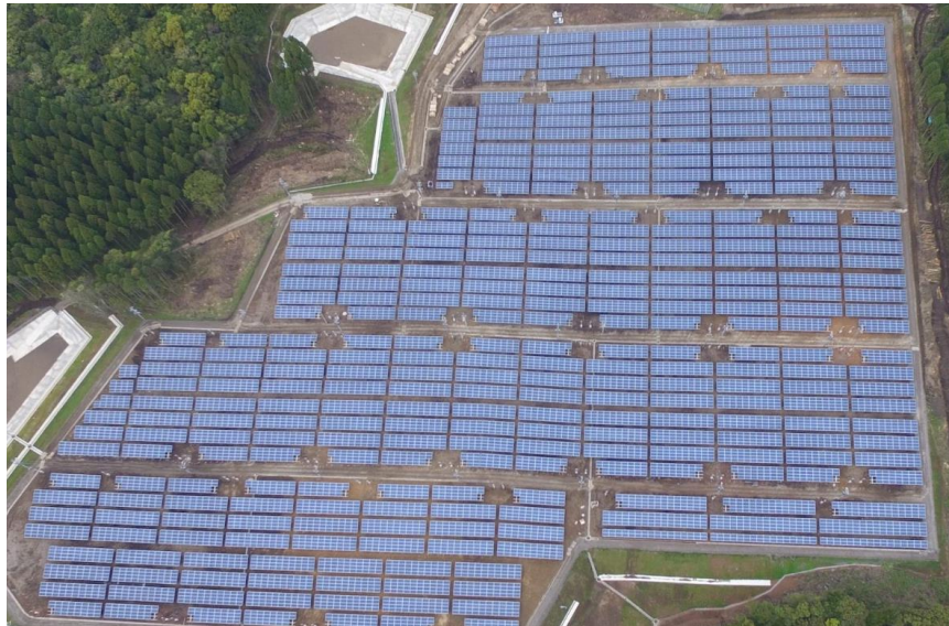
Miyanoura Solar Power Plant (Kagoshima Prefecture) / (DC): Approx. 2.8MW
