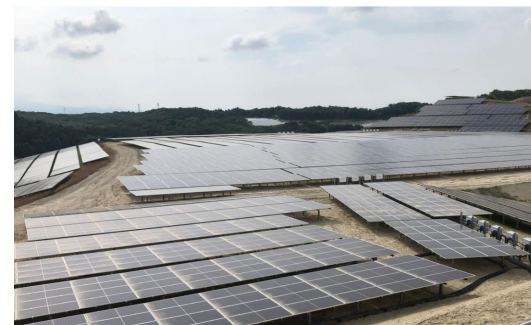
Taiwa Town Solar Power Plant/ (DC) 10.8MW
